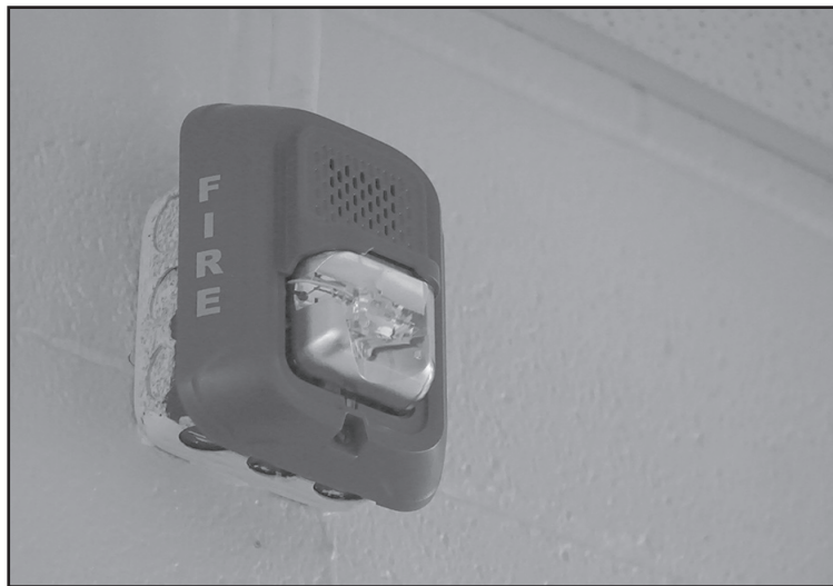
A fire alarm in Coronado Hall is shown Tuesday. Students have voiced concerns about fire alarm malfunctions throughout the school year.
