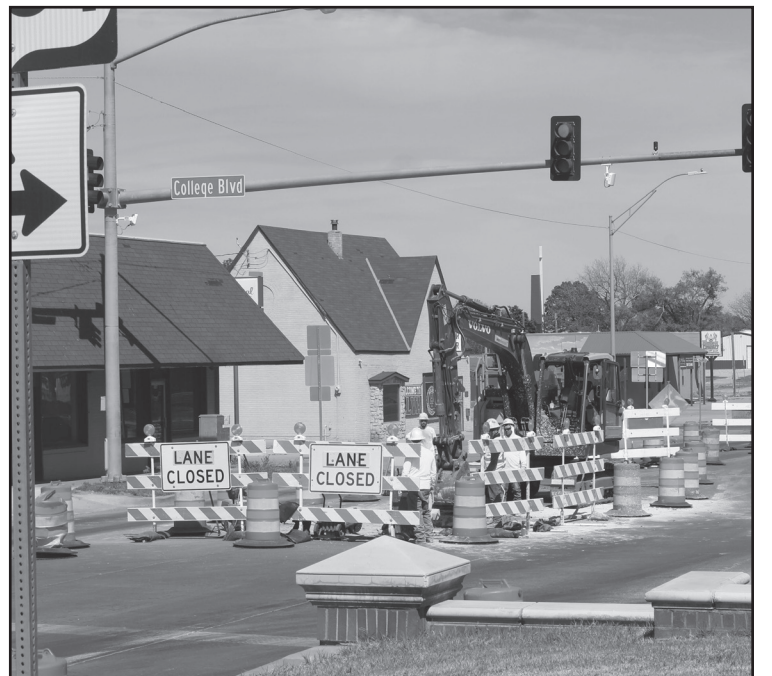
Workers digging a hole in the middle of the road as they prepare their construction work to upgrade the water system in town which is causing traffic jams on College Blvd.
