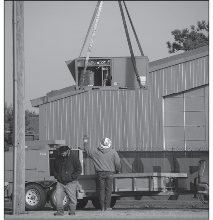
Photo by Ingrid Maldonado Workers replacing air conditioning unit at Percefull Fieldhouse causing classes to be moved out of the Health and Sports Science Building.
